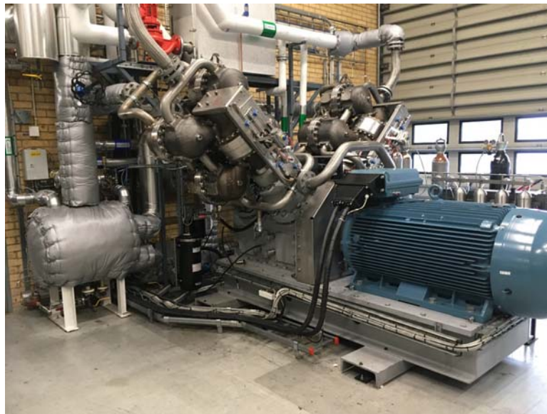
Fig. 1. The HighLift Stirling-cycle-based heat pump (SC HP) from Olvondo Technology is installed in the heat pump room at pharmaceutical company AstraZeneca, Gothenburg, Sweden. The nominal heat output from the heat pump is between 450 and 500 kW [6].
